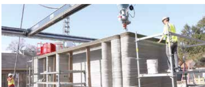
A 12-ton industrial 3-D printer is used to print concrete two-story home
